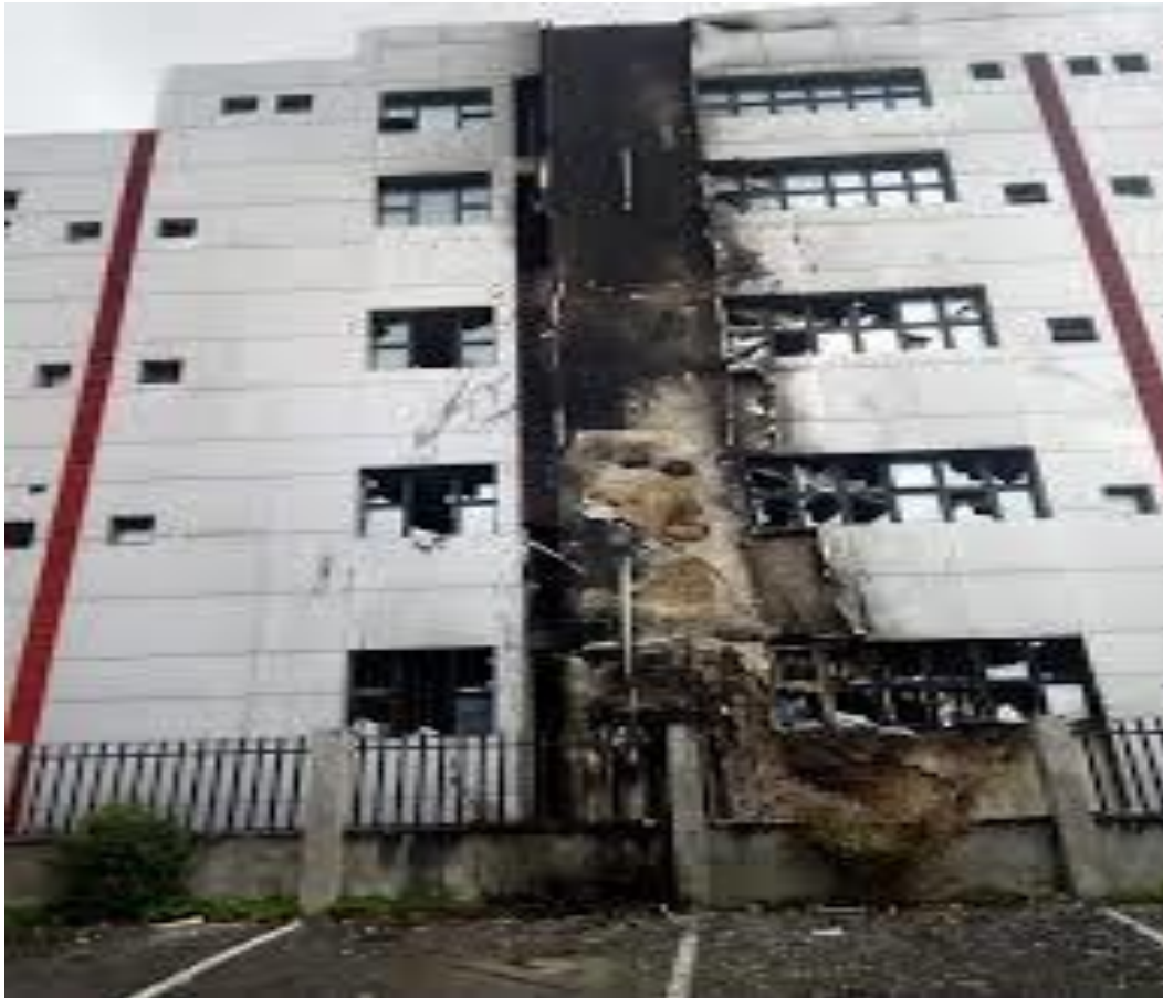
Figure: 4 State Secretariat of the All People Progressive Party, Destroyed By Fire. Source: Field work (2025)
