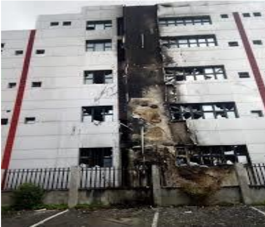
Figure: 4 State Secretariat of the All People Progressive Party, Destroyed By Fire. Source: Field work (2025)
